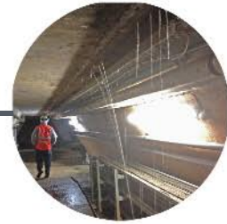
Leaking bridges, tunnels and basement structures
