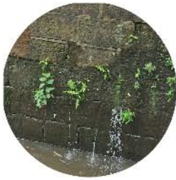
Leaking retaining walls
